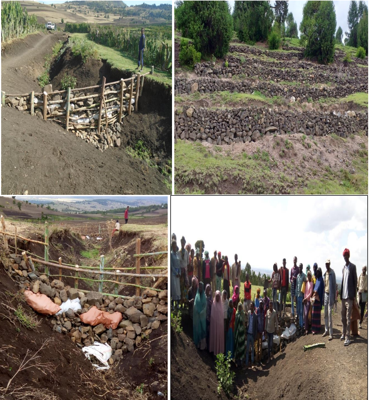
Figure 4: Picture during community-based participation in implementing soil and water conservation structures in Ilasa watershed
